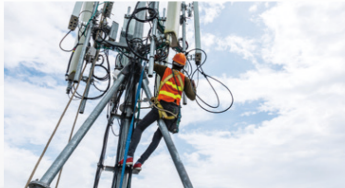
Lone worker protection services
