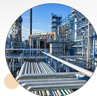
D Monitoring leaks and other disruptions in processing plants
